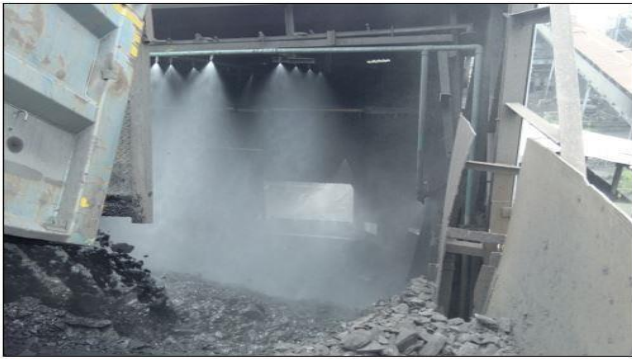
Automatic sensor based mist spray system arranged at coal receiving hopper of CHP.
