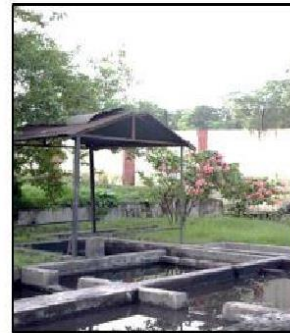
Oil and grease tank
